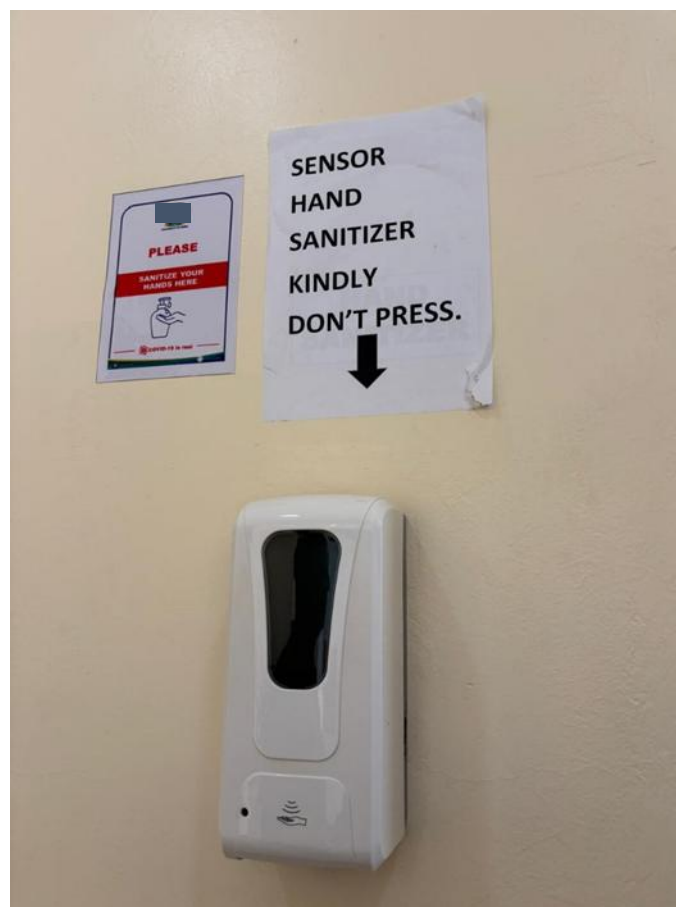
Figure 3: An empty wall-mounted sanitizer dispenser in a hospital corridor. The dispenser remains attached to the wall but is no longer refilled, marking the withdrawal of institutional maintenance
